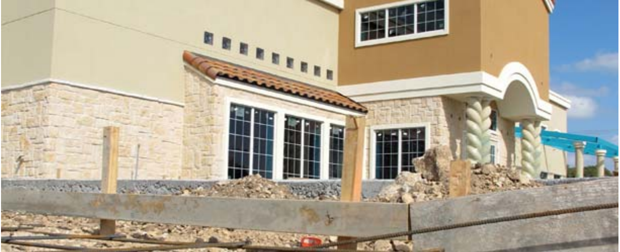
Sidewalks and parking lots are the finishing touches for new tenants in 1890 Ranch like Rosa's Cafe, Cedar Parks newest Mexican Restaurant. Photo by GREGG CESTARO
